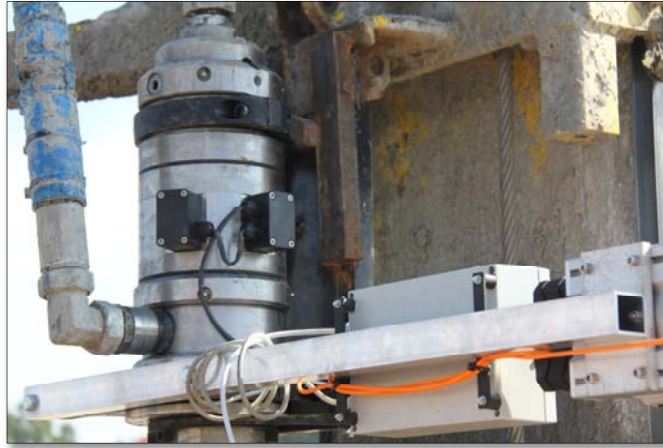
Fig. 7: Inlet of electric current into the drilling rod
